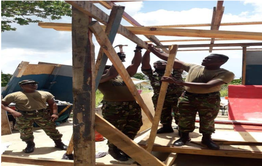
Photo 1: Members of the Trinidad and Tobago Defence Force 1 ST Engineering Battalion support the reconstruction of homes in the Rousillac Village, Siparia following severe weather.
